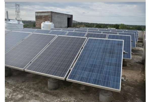
Solar Power Facility
